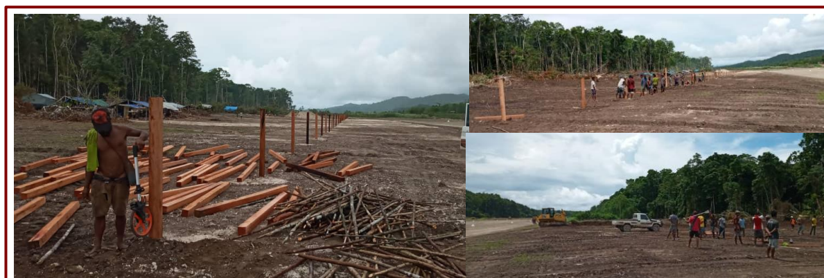
Six hundred (600) youths of Esa'ala District engaged in the clearing and upgrade of the Miyadeba Airstrip, working closely with the civil engineers, Esa'ala District, Milne Bay Province, 2020
